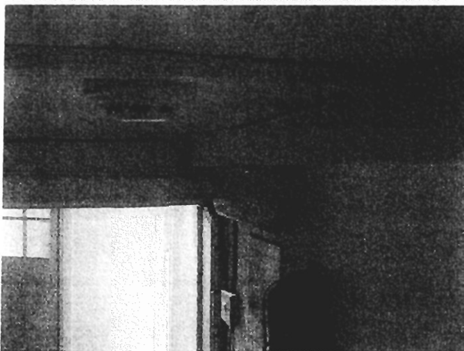
Smoke Detector and Non Maintained Emergency Light plus Floor Plan
