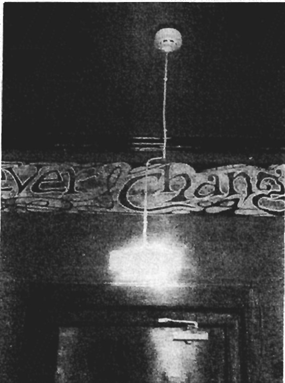
Maintained emergency Light and Smoke Detector, 2nd floor room
