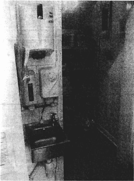
Ice Machine removed, dry store only
