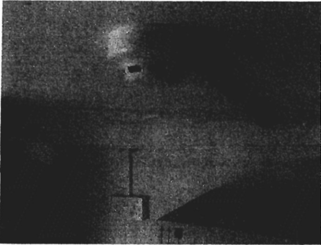
Smoke Detector and Spare Sockets
