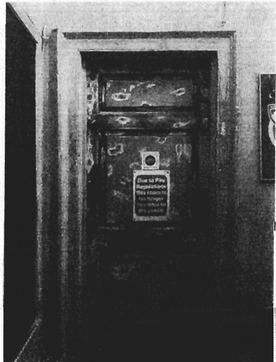
2nd Floor room closed, keypad and now Fire Door
