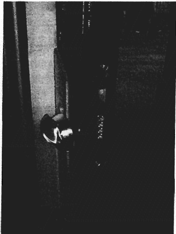
Current Fire lock on front door, there are 2 of these
